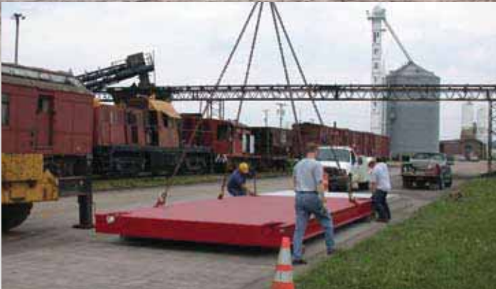
Module A is unloaded from the truck and placed on the foundation.
